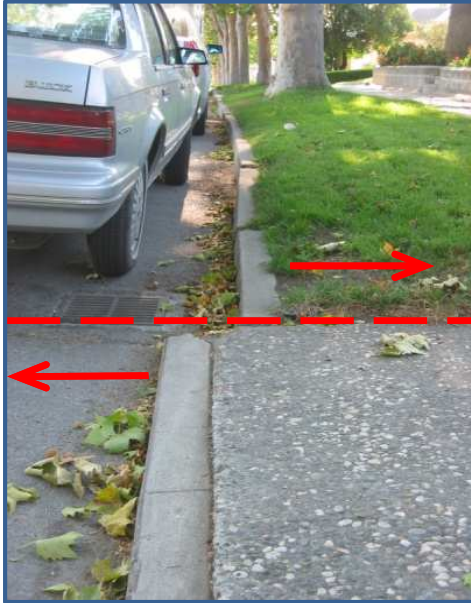
Right-lateral offset of curb at 6 th Street near Dunne Park
